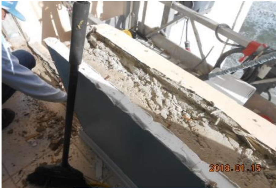
Original wet-set concrete at sill seen after window collapse in Unit 2103
