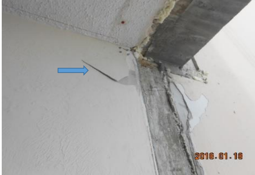
Delaminated plaster inboard of window opening, Unit 2103 guest bedroom
