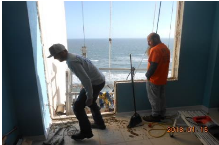
Sill repair work in progress at east guest bedroom window in Unit 2103
