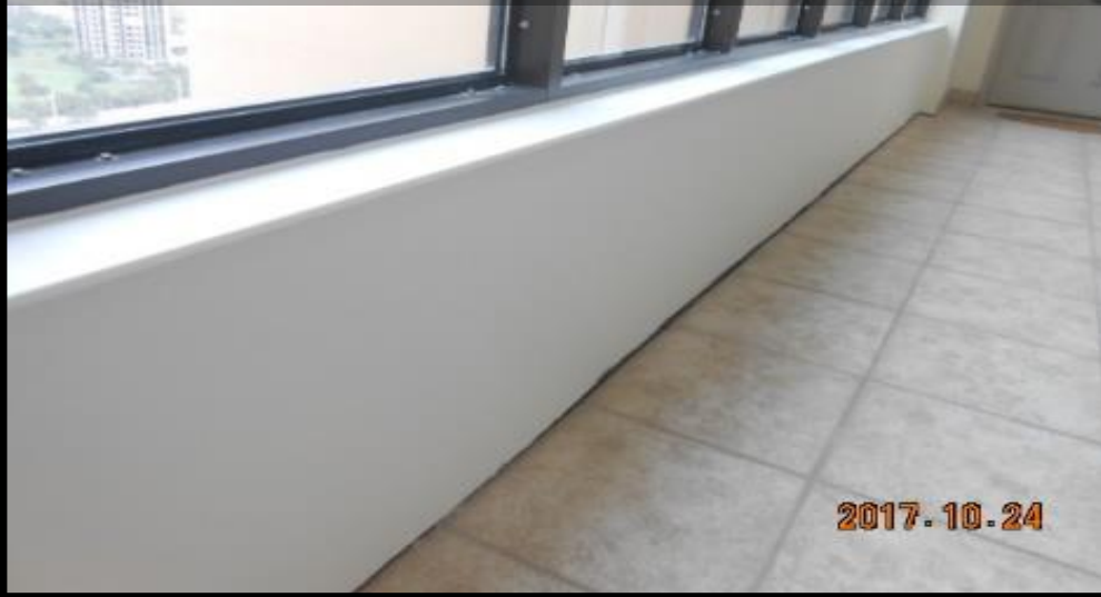
Finished and painted interior knee wall with Corian sill mockup installed at the penthouse floor
