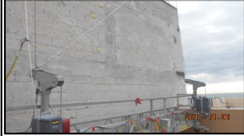
Stucco stripped down to masonry at center shearwall at roof level
